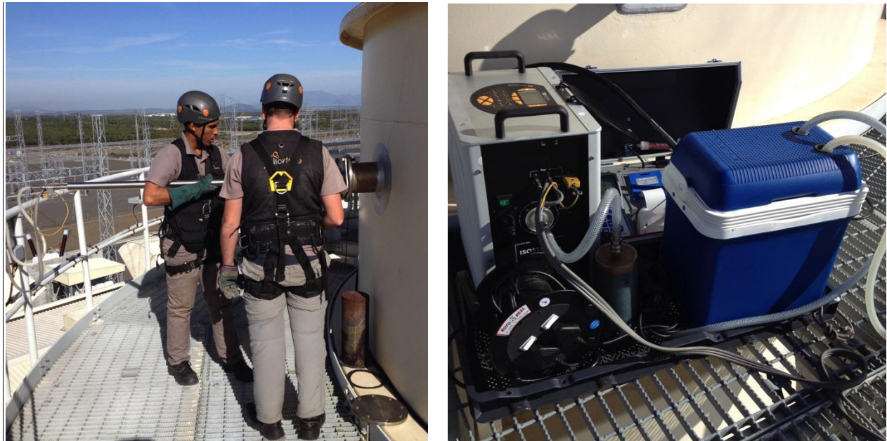
Figure 2: Yellow Tree's Testing Equipment
